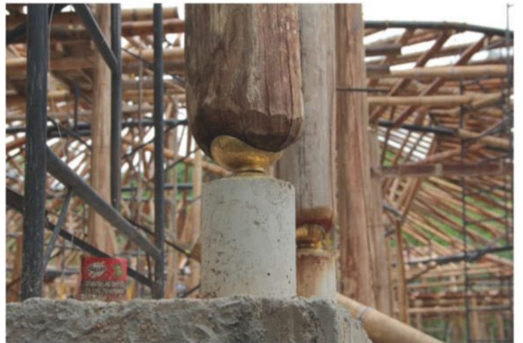
Opposite, top: Close-up view of the adjacent pavilion's roof structure. Opposite, bottom: General view of the pavilion. This page, clockwise from top right: Pavilion during construction. Detail of the joint between column and foundation. Details of the pavilion's roof joint using bamboo rhizomes. Details of the roof joints on the main house.
